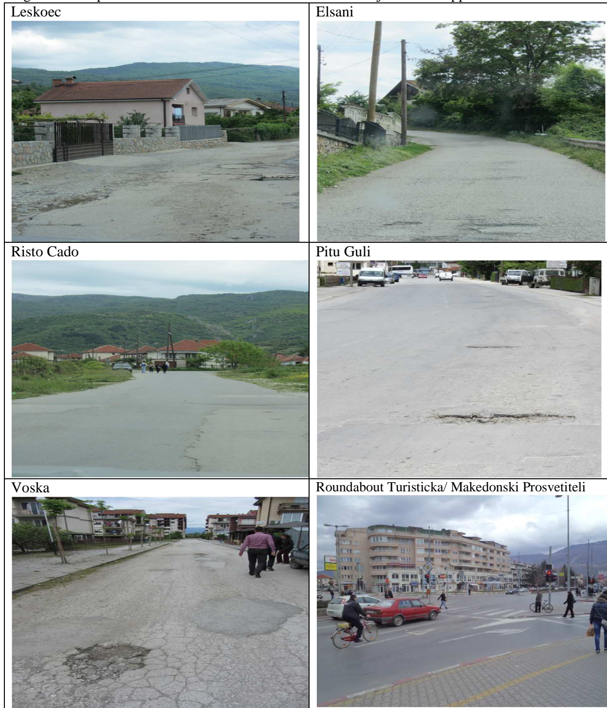
Figure 3: The present condition of the local roads/streets subject to this appraisal
