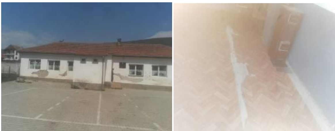
Figure 1. Pictures from the current situation of elementary school in the settlement of Cerovo
